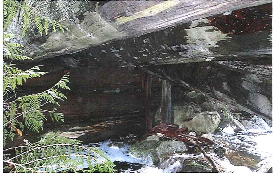
CK2178 Failed Stringer
